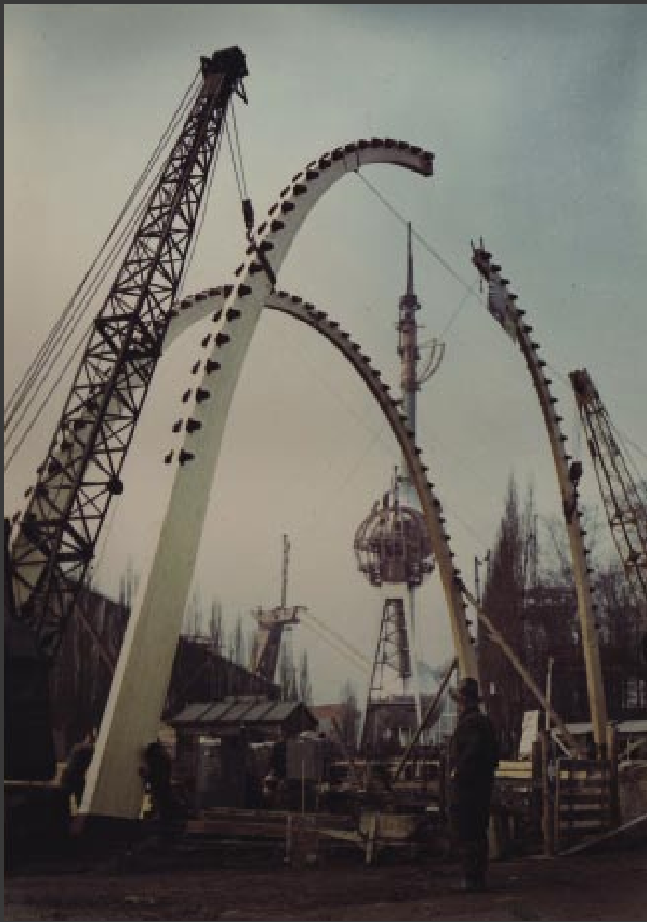
Construction of the Expo 58 cable-car with beams by De Coene, design by Roger Thirion ARCHIVE STICHTING DE COENE VZW
